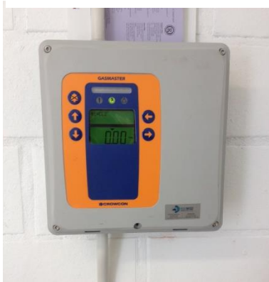
Chlorine Leak Detector Control Unit
