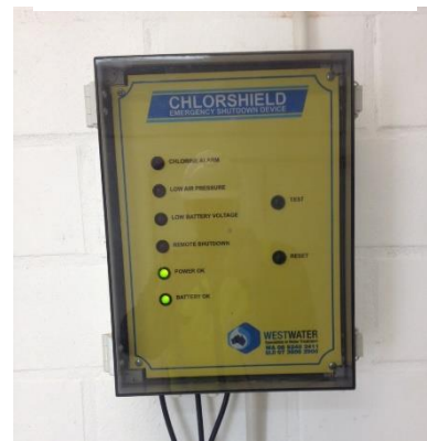
Emergency Shutdown System Control Unit
